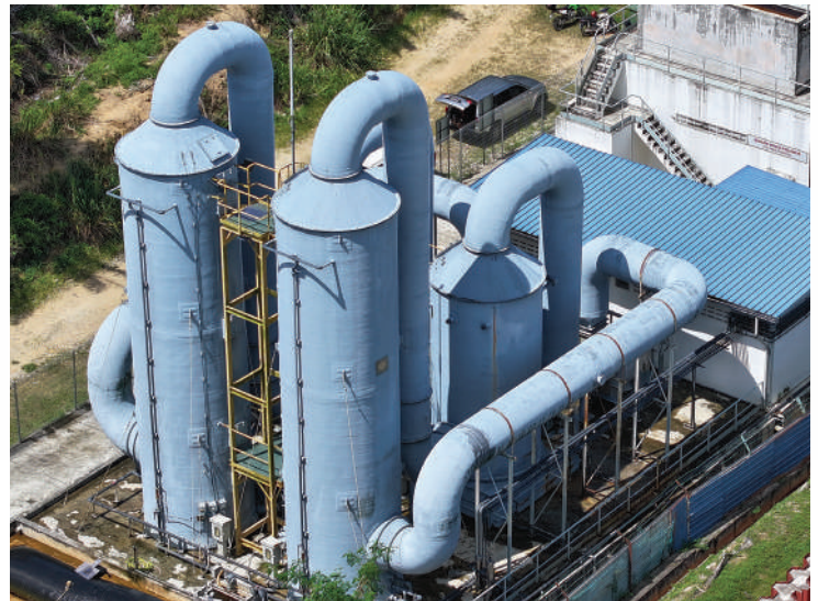
Pollutant Removal System, Simpang Renggam, Johor
