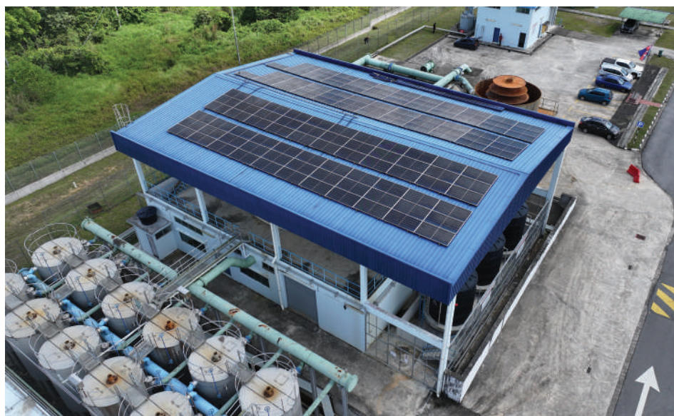
Ranhill's 63 kWp Solar PV System at 20 MLD Sultan Iskandar WTP
